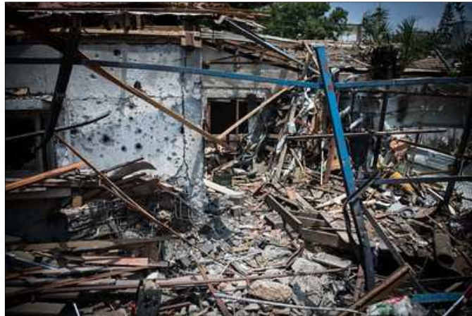
House destroyed by Hamas rocket, Yahud, Israel, July 22, 2014. Most often, whenever the Jewish state responds in strength to acts of aggression, it is chastised for “disproportionate use of force.”
